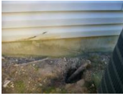
hole in soil seems to drain under house. Also note siding damage
