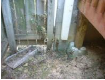
Downspout needs extension. This water wall has cause deck support to settle
