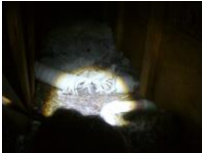
damaged vent pipe (behind furnace in attic)
