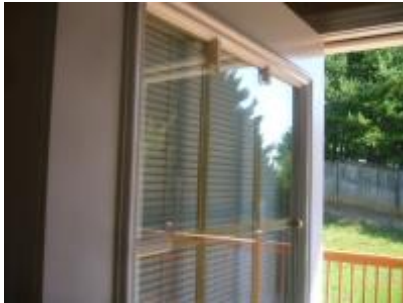
rear exit door to deck. Grill broken
