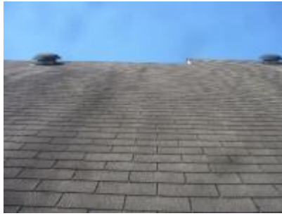
rear roof deck. note two power vent fans
