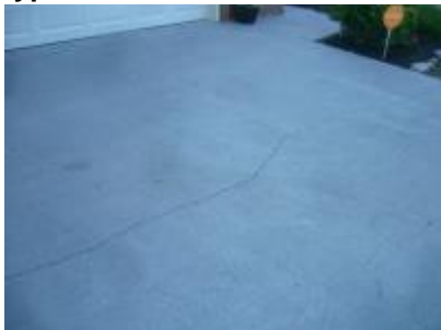
crack in upper slab
