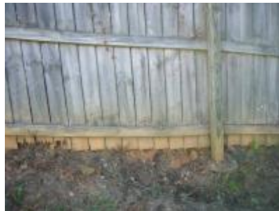
fence boards damaged at bottom
