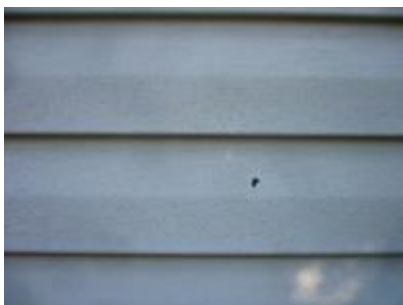
Small siding hole, right rear corner of house
