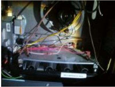
interior of attic furnace
